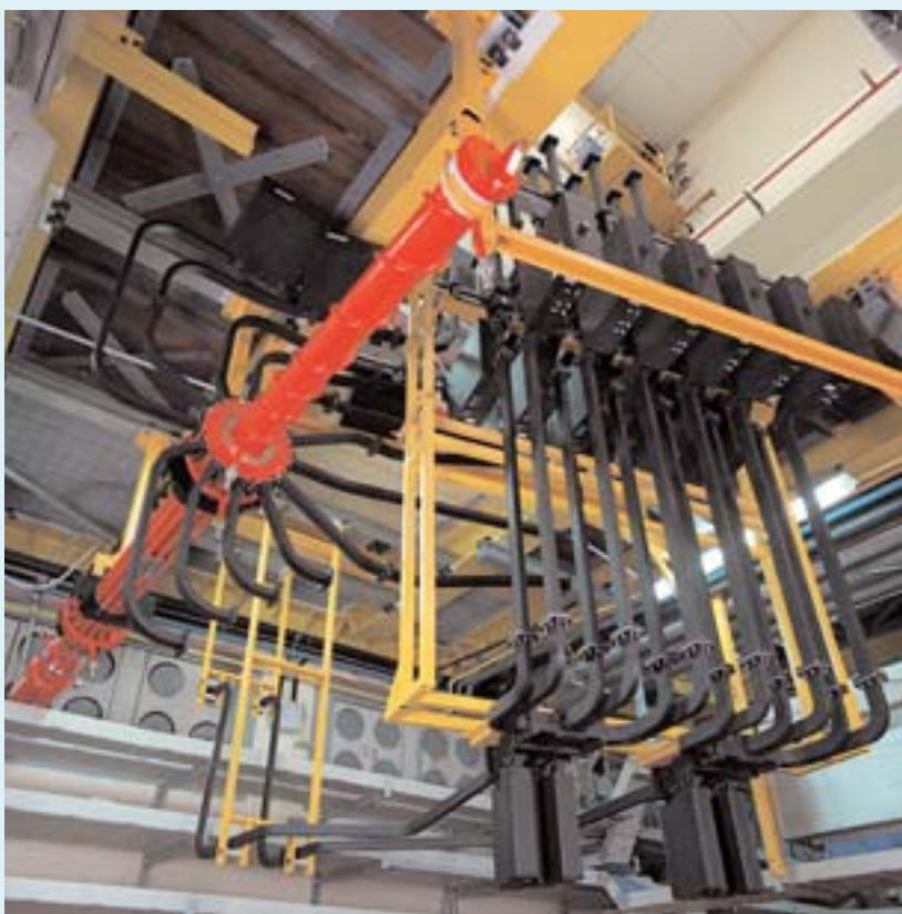
End converter of main transmission line to the 12 LHCD waveguides of FTU
